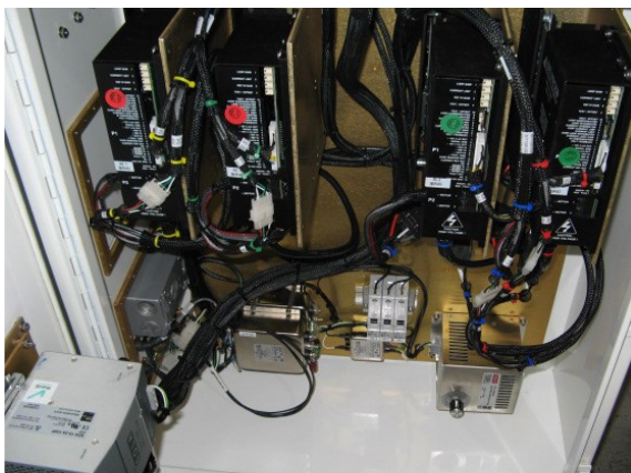
The Pedestal Interface Unit (PIU) contains all of the pedestal electronics.
